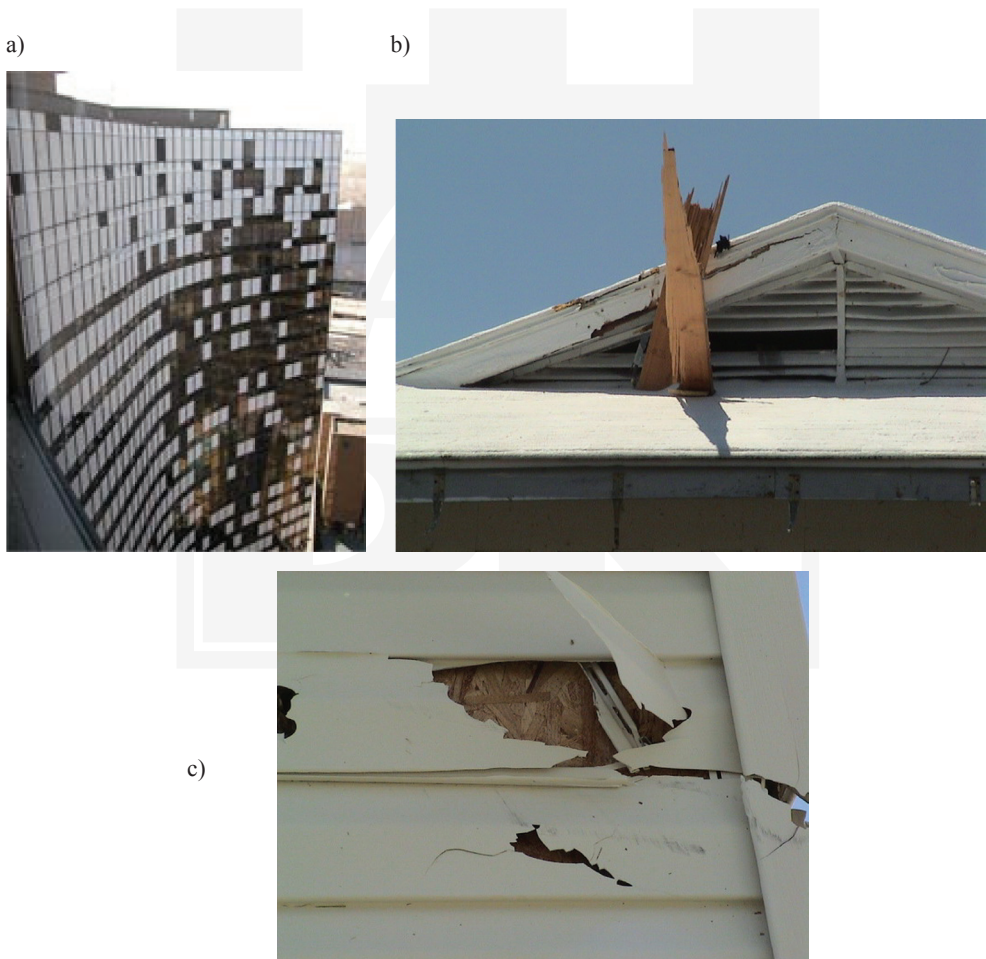
Fig. 1. Examples of damage caused by windborne debris, a) north façade of Hyatt Hotel, New Orleans damage by pea gravel from neighbouring roof (photo by K. Porter for MCEER), b) example of hazard due to missiles generated by failed structures (photo by T. Reinhold, AAWG gallery), c) example of cladding damage due to windborne missiles (photo by T. Reinhold, AAWG gallery)
