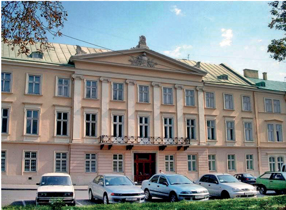
Fig. 20. Polychrome façade scheme in Classicism – light yellow background, white details (Vynnychenka Str.) (Photo by A. Kazantseva)
