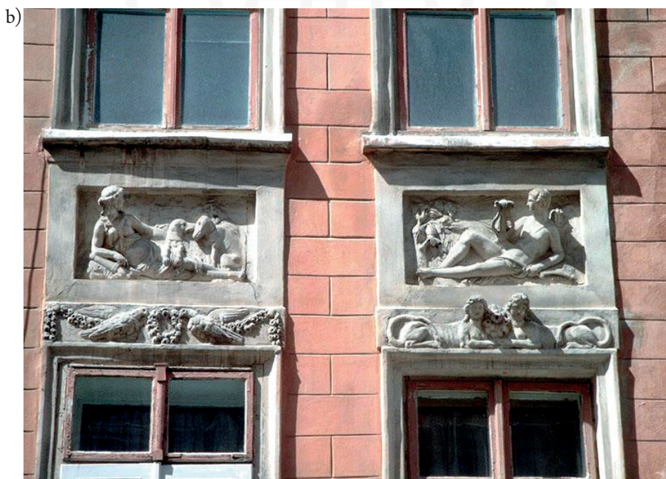
Fig. 22. Colouring façade scheme in Empire Style: a) black background of bas-reliefs (26 Krakivska Str.); b) red façade background (10 Shevska Str.) (Photo by A. Kazantseva)
