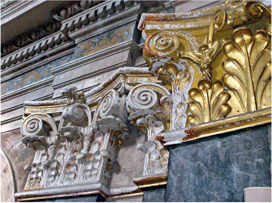
Fig. 17. Traces of red support base under gilding, Jesuit Church (Photo by A. Kazantseva)
