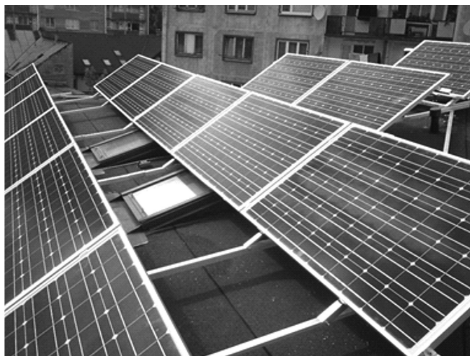
Fig. 1. Installed photovoltaic system
