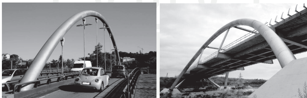
Fig. 1. Structural use of stainless steel in road viaducts and bridges: Arco di Malizia, Siena, Italy (left) and Piove di Sacco Bridge, Padoa, Italy (right) [1]
