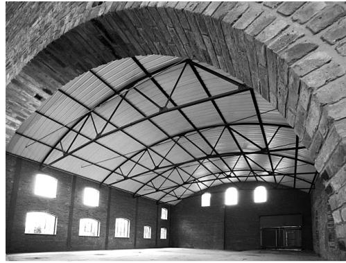
Fig. 14. The interior of the workshop part of the former gas plant, with its characteristic construction of steel girders added at the end of the nineteenth century (source: [31])
