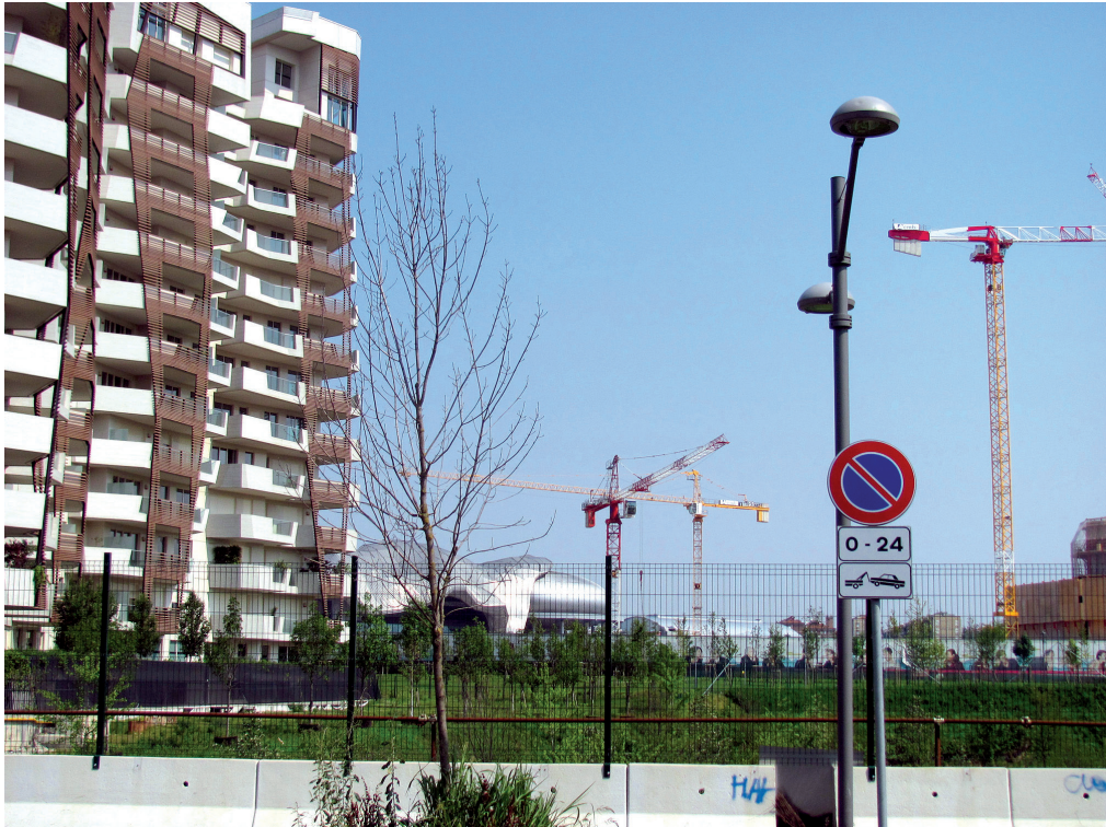
Fig. 8. Milan, part of a fenced and guarded complex of residential buildings 'City Life', under construction. The buildings visible in the picture have been designed in the studio of Daniel Liebeskind (photo by K. Dudzic-Gyurkovich)
