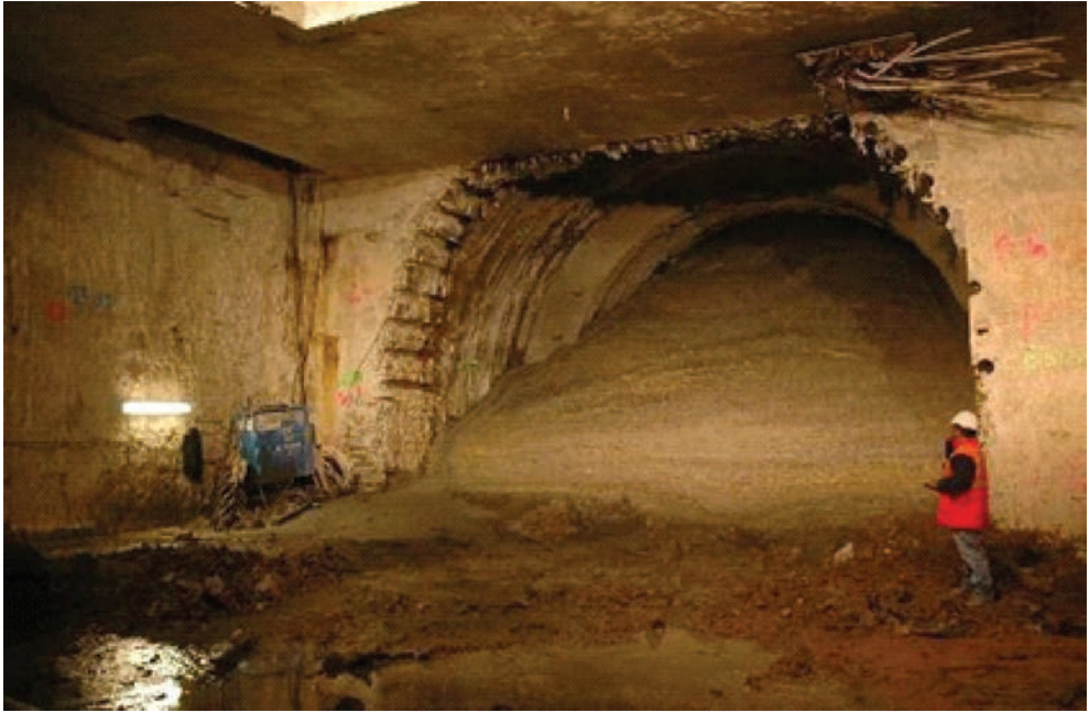
Fig. 5. Initial phase of soil liquefaction after the heave of excavation work ceiling [11]
