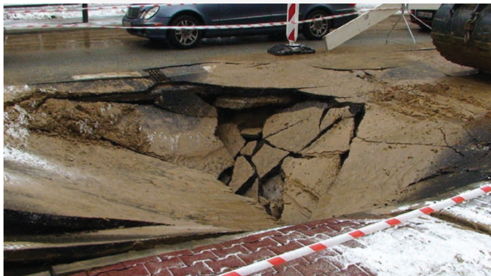
Fig. 3. Subsidence on Koszykowa Street in Warsaw (source: TVN24 publication)
