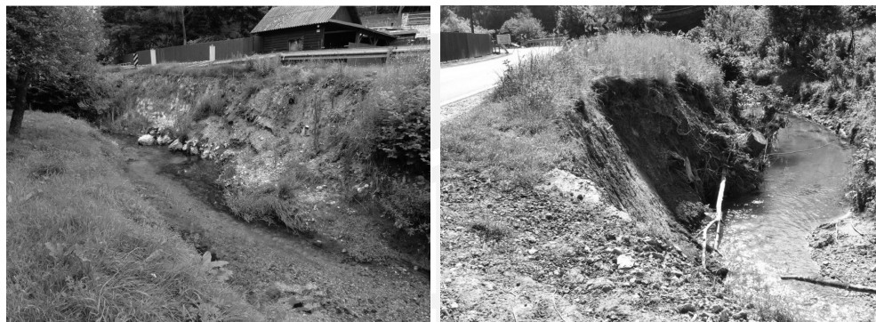
Fig. 1. A damaged fragment of the fill slope and the Prądnik (Białucha) stream undercutting it (Source: [5])
