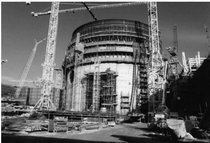
Fig. 3. Execution of Reactor Bldg. in Sizewell B power plant (photo by K. Tracz)
