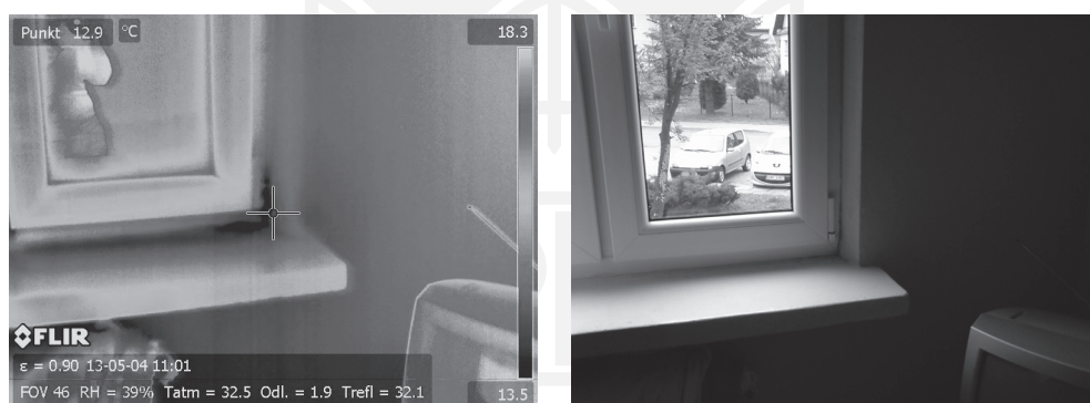
Ill. 8. Thermal bridge – connection between window jamb and external wall in building number 1
