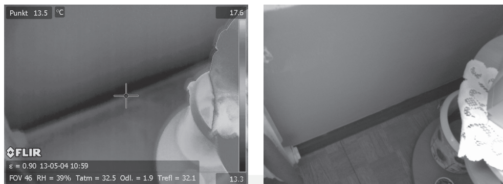
Ill. 7. Thermal bridge – connection between floor and external wall in building number 1
