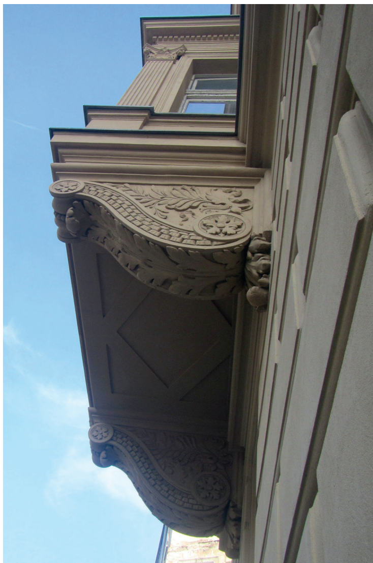
III. 4. Status after conservation work at townhouse at ul. Studencka 14 in Kraków, detail of a bay window in the south-western façade from the side of ul. Garncarska
