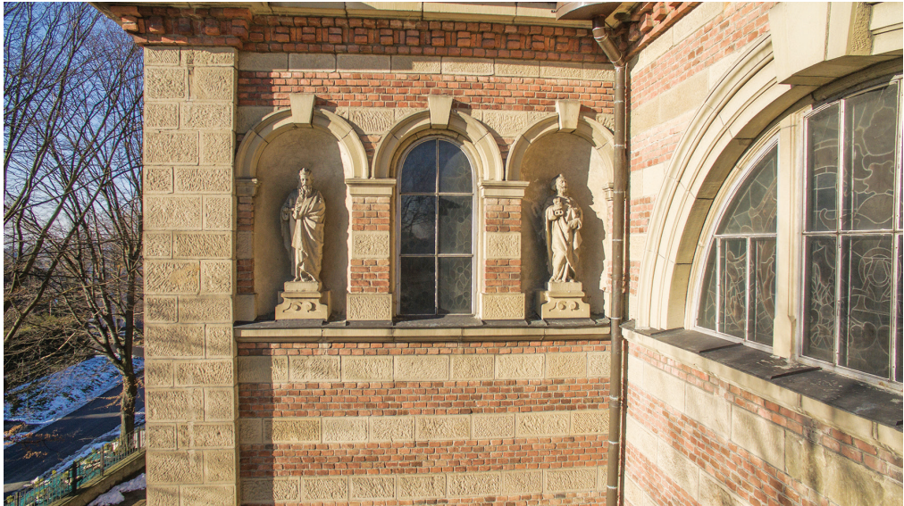
Fig. 3. Parish church in Mystkow – façade details
