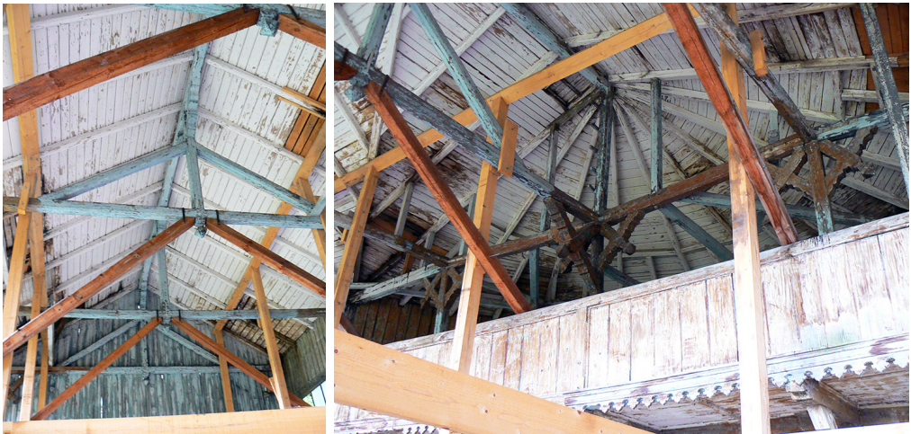
Fig. 8. Interior of the middle segment - view of the western wall - the open roof truss, single-frame with struts and king posts supporting the ridge. A view of the interior of the avant-corps – the closed balcony balustrade, the avant-corps roof truss and secondary reinforcement of the original structure are visible. This is the condition before the adaptation of the pavilion (Source: Author's archive)
