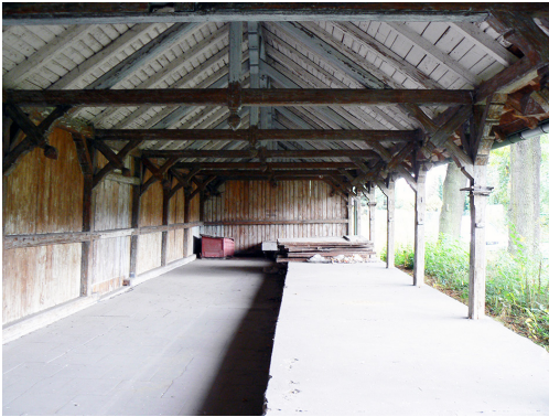
Fig. 6. View of the eastern segment interior eastwards; on the left and in the background there are the walls with a half-timbered structure, on the right there are posts of the open wall of the hall immersed in a concrete shooting bench (post-war) – the other side presents the original level of the hall (concrete pavement slabs, possibly from the inter-war period). This is the condition before the adaptation of the pavilion (Source: Author's archive)
