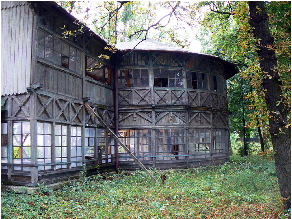
Fig. 9. The critical condition of the shooting range pavilion showing a view of the central section from the southern side. This shows the condition before the adaptation of the pavilion (Source: Author's archive)
