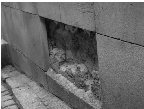
III. 7. Sandstone plinth. Eroded slab due to water vapour condensation, Olomouc, The Czech Republic
