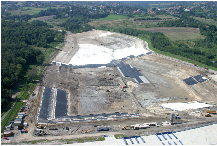
Fig. 14. Municipal landfill construction on the Central Field (from archive Salt Mine “Wieliczka”)
