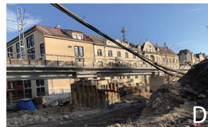
Fig. 10. Selected fragments of the area, two overview photos: zone C – historic viaduct at “Grzegórzki” junction and new-built flyover situated along existing market Unitarg, lower photo: zone D – view of the flyover along Blich St. (by E. Komarzyńska-Świeściak)
