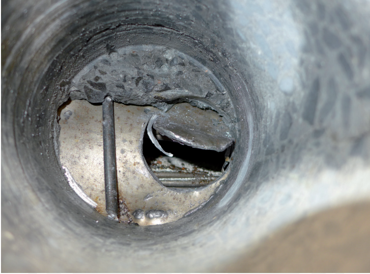
Fig. 4. View into the drilled hole in the girder subjected to investigation. The steel cover of the prestressing cable duct and its interior are visible
