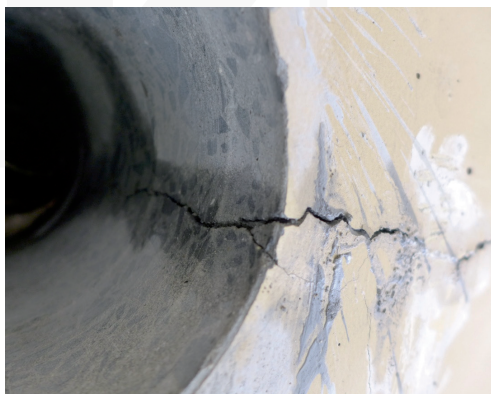
Fig. 3. Crack position in the drill wall of the beam under investigation
