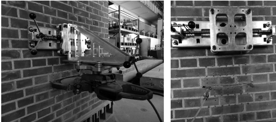
Fig. 3. High precision slot cutting using the RING type circular saw and designer stand (on the left) and view of the wall during the flat jack test (on the right)
