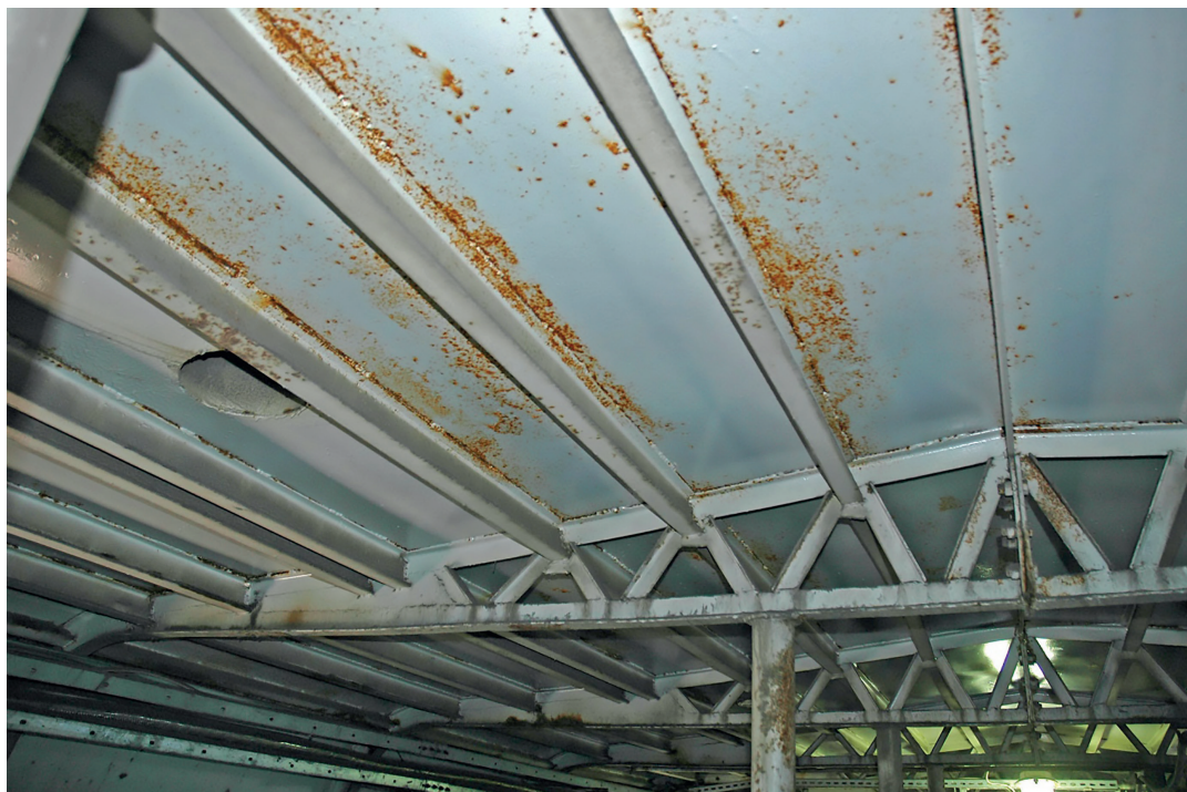
Fig. 4. Interior of the gallery – visible fragment of the roof section – steel structural elements and sheet metal
