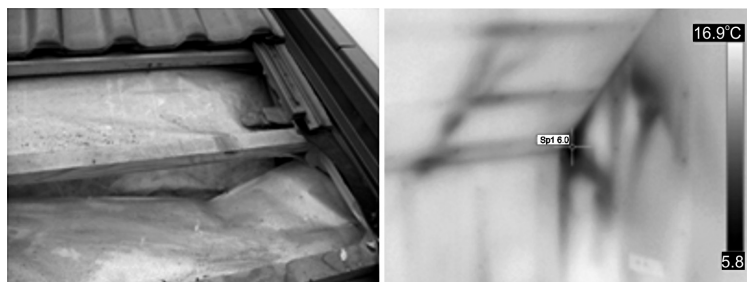
Fig. 1. Picture of poorly constructed roof and corresponding thermogram illustrating the impact of one-sided ATBs on heat transfer. Interior temperature t_i = 18^\circ\text{C} , exterior t_e = -10^\circ\text{C}
