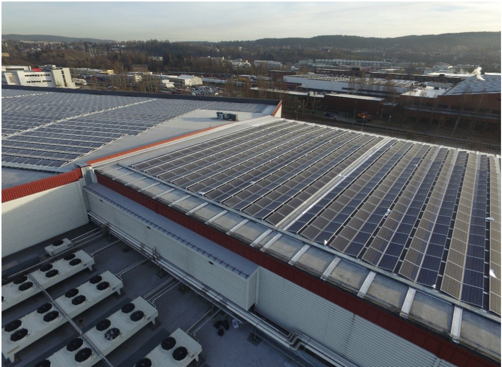
Fig. 1. The Weight Watcher system installed at the warehouse
