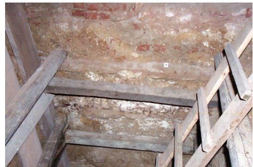
Fig. 14. A deep excavation confirming the lack of a basement in this part of the building (source: [31])
