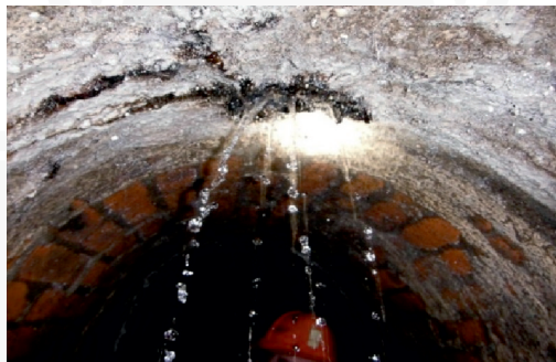
Fig. 5. Leakage into the collector (source: [13])
