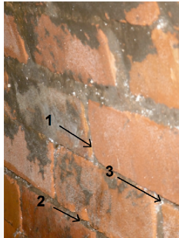
Fig. 4. The wall of the collector. No 1, 2, 3 are places of mortar loss (source: [13])
