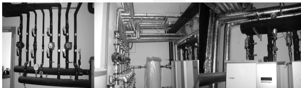
Fig. 2. Heating installations 4 heat pumps brine-water used for heating, ventilation and air-water heat pump for domestic hot water needs
