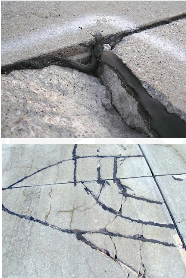
Fig. 1. Damaged expansion gap filled with bitumen
