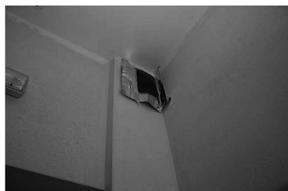
Fig. 8. Loosened sealed opening during the airtightness test
