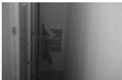
Fig. 7. Loosened sealed opening during the airtightness test
