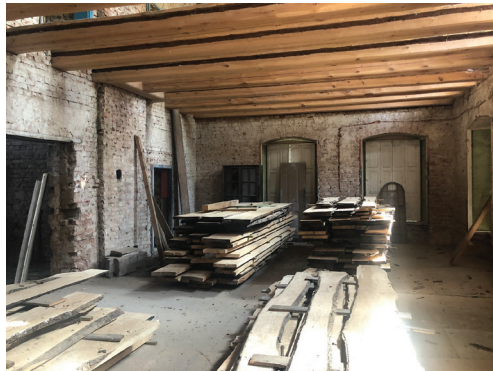
Fig. 5. Rychnów (dep. Namysłów), palace, ground floor, hall in front of the eastern crosswise sections, present state (photo by A. Legendziewicz)
