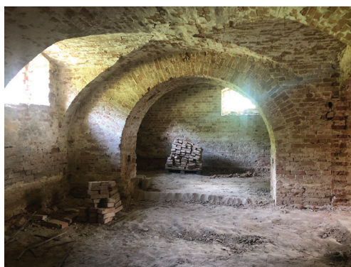
Fig. 9. Rychnów (dep. Namysłów), palace, basement, back chamber in the eastern crosswise sections, present state (photo by A. Legendziewicz)
