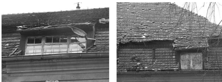
Fig. 12, 13. The condition of roofing and guttering before renovation, 2008
