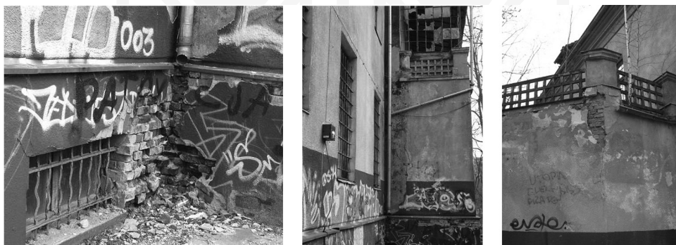
Fig. 14–16. The damage to walls caused by soaking, 2008
