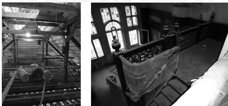
Fig. 8, 9. The timber roof structure and the view from the entresol over the two-storey fireplace ballroom with stained glass windows, 2011
