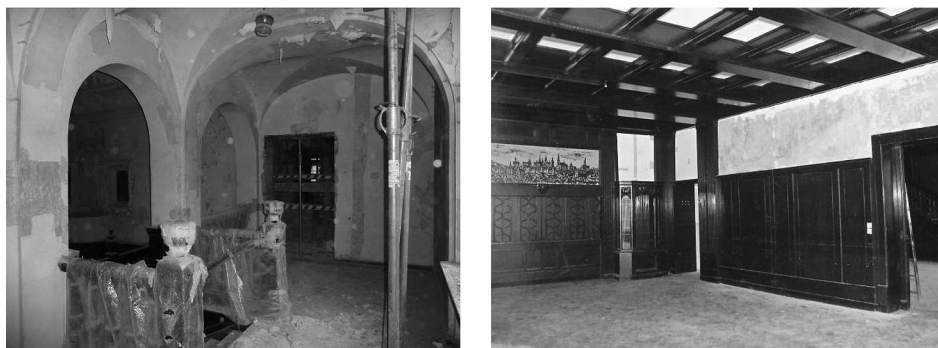
Fig. 6, 7. The groined vault covering the entresol in the fireplace ballroom and a coffered ceiling above the dining room on the ground floor, 2011
