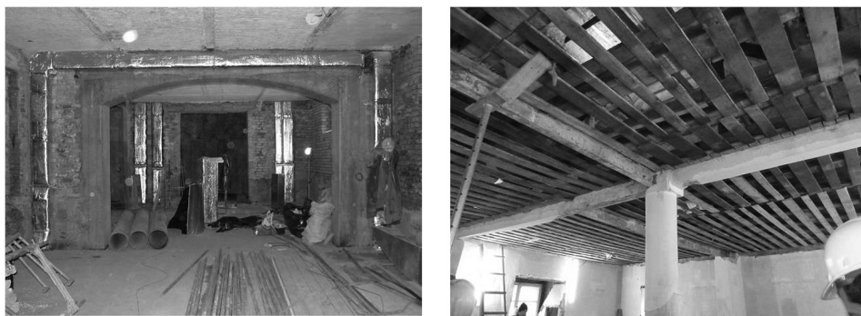
Fig. 4, 5. The brick ceiling above the basement and the timber ceiling (above the attic) supported by steel binding joists and a steel column, 2011
