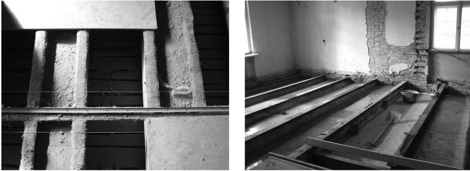
Fig. 23, 24. The timber ceiling beams strengthened by additional wooden elements from both sides, and a new R-C ceiling based on steel beams, 2011
