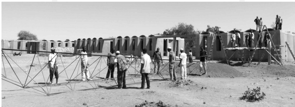
III. 9. Lower secondary school in Gando. Burkina Faso. School building during construction (source: [6])
