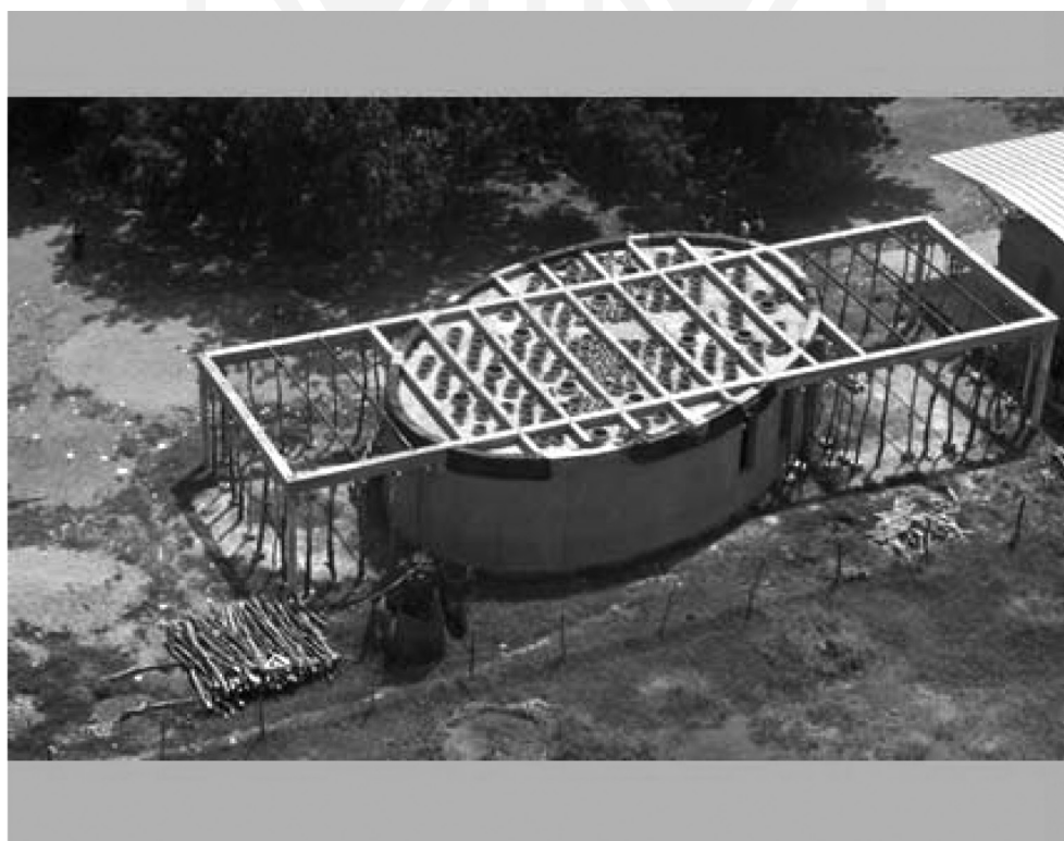
Ill. 14. Library in Gando. Burkina Faso. Top view of a ventilated roof (source: [2])
